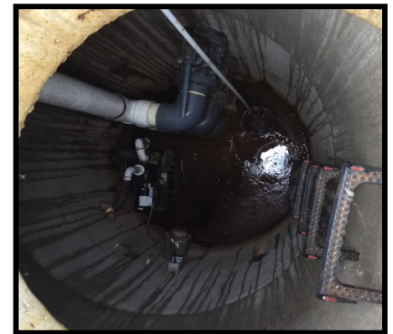
Confined space in a manure storage system
